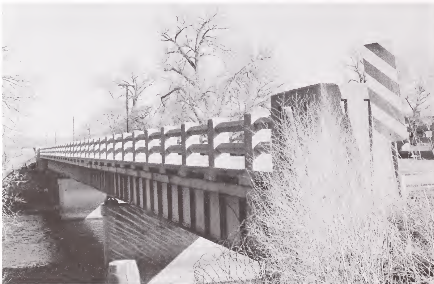
Clark's Fork of the Yellowstone River Bridge north of Belfry. The structure was fabricated by the American Bridge Company and built by Miles City contractor Jerome Boespflug in 1939.
